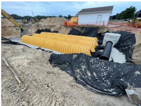
North Underground Detention System
