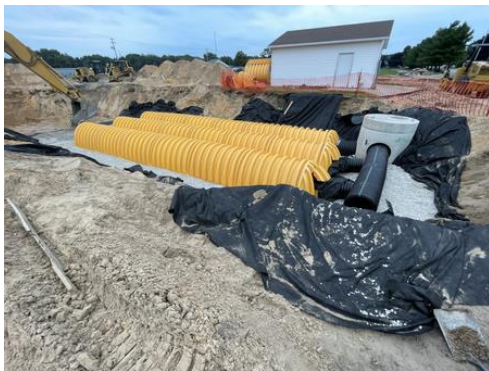
North Underground Detention System
