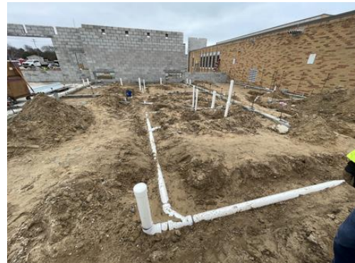
HS Office Underground Plumbing
